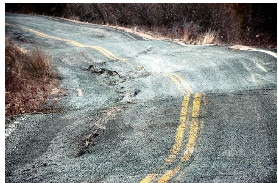
Figure 2: Damaged roads due to permafrost in Canada.
